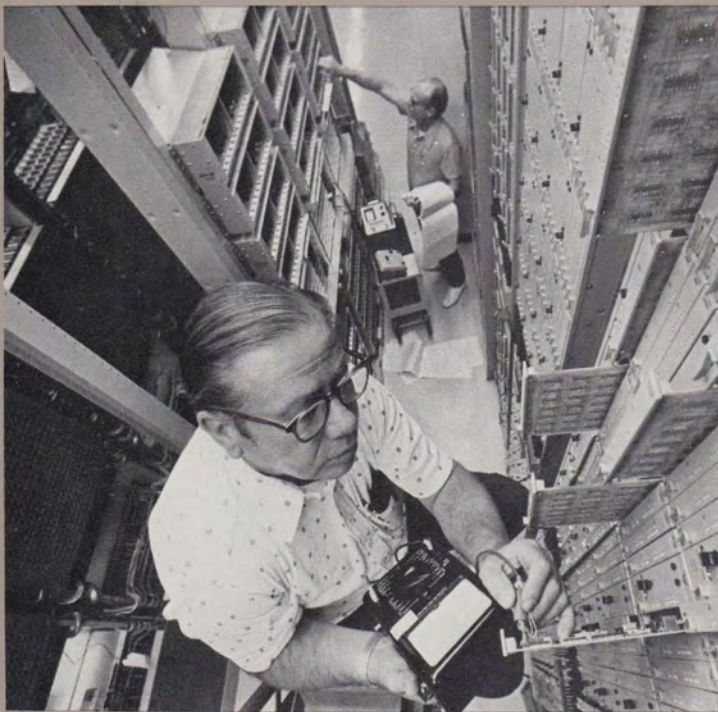
Bird's eye view of the first installation of T-1 Carrier, a digital or pulse-code modulation system for transmitting signals on inter-office trunks largely in urban areas.
